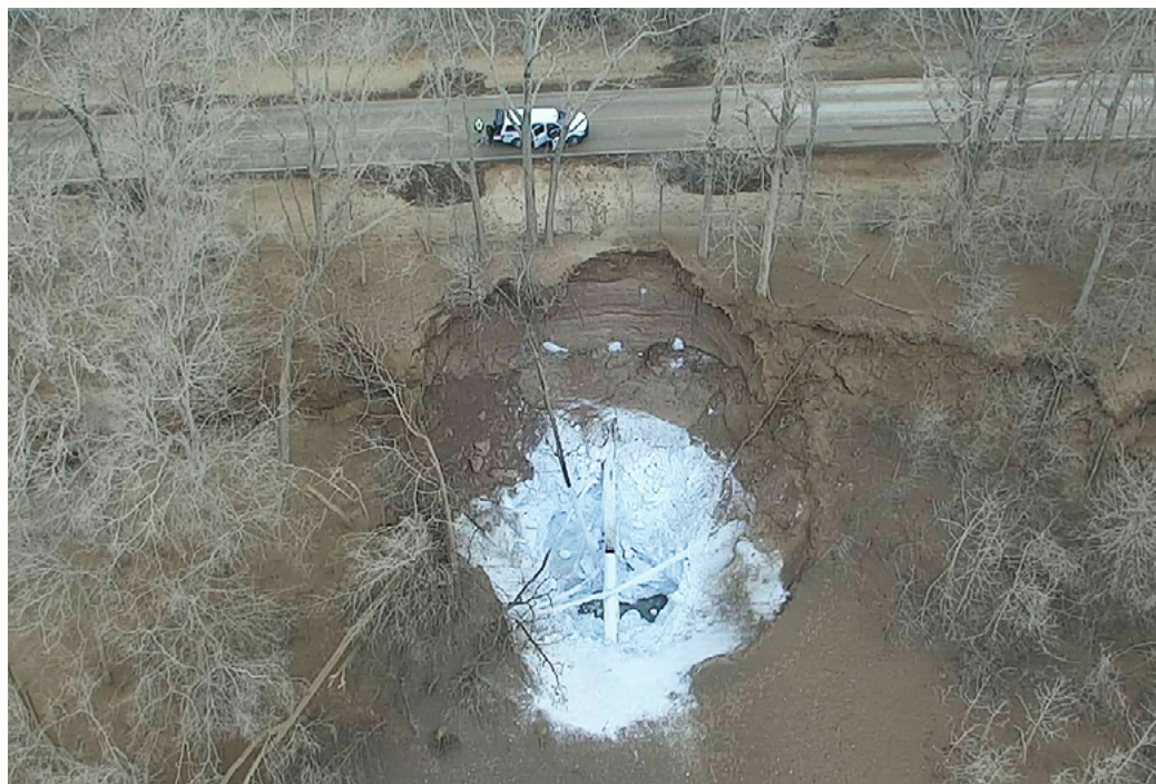
Figure 6. Aerial Drone Photograph of Satartia, MS, Denbury Pipeline Rupture.
